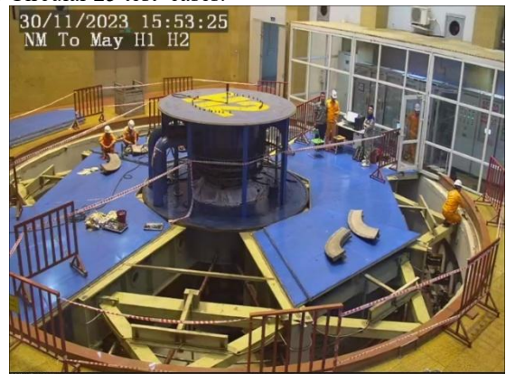
Figure 11: Ban Ve hydropower generating unit during preparation for field testing
